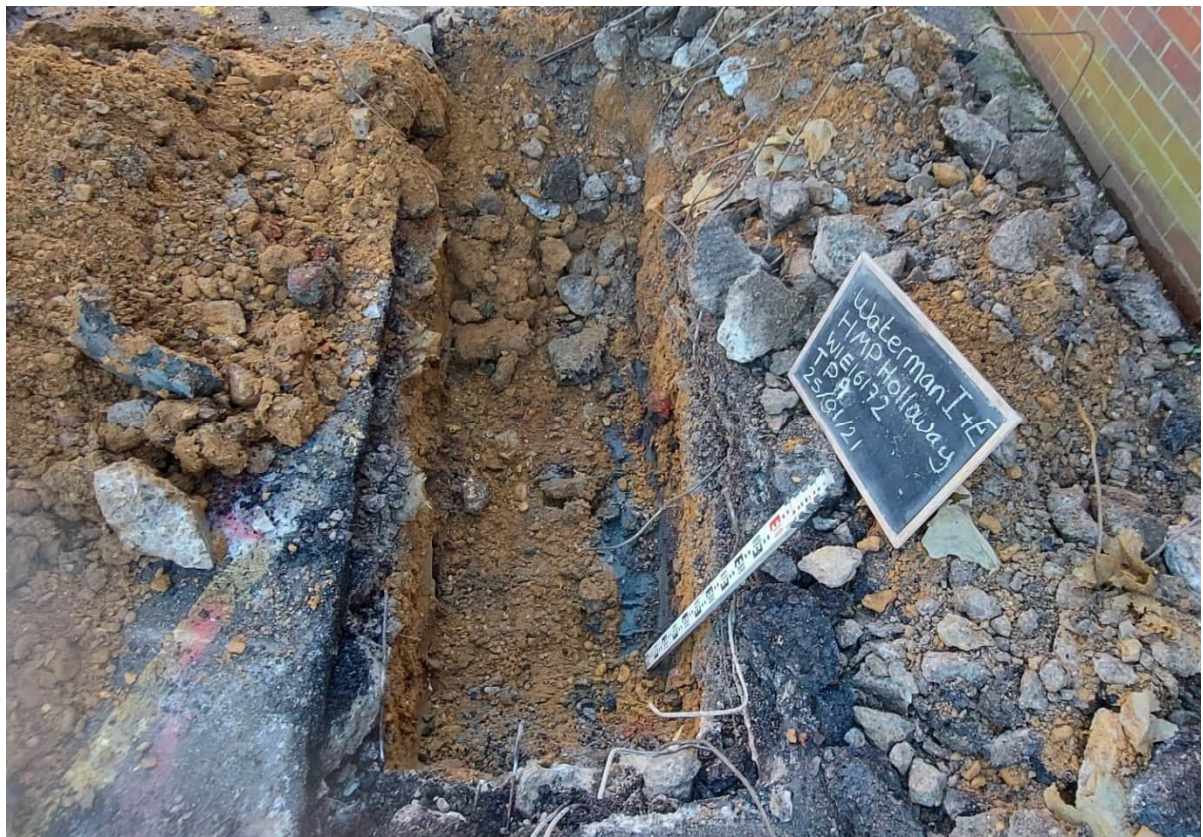
Photograph 10 – TP09 with staining visible along the southern face of the pit.
