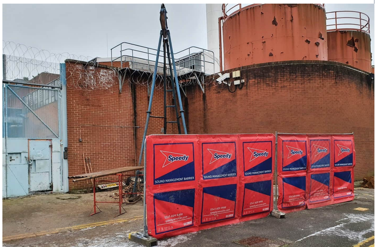
Photograph 3 – Pilcon 1500 cable percussive drilling rig in position over BH02 with acoustic barriers in place.
