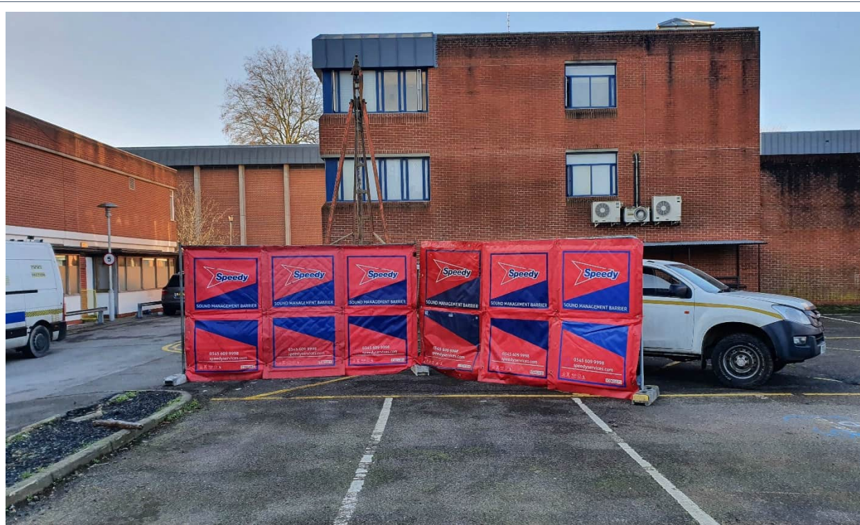
Photograph 2 – Dando 3000 cable percussive drilling rig in position over BH08 with acoustic barriers in place.
