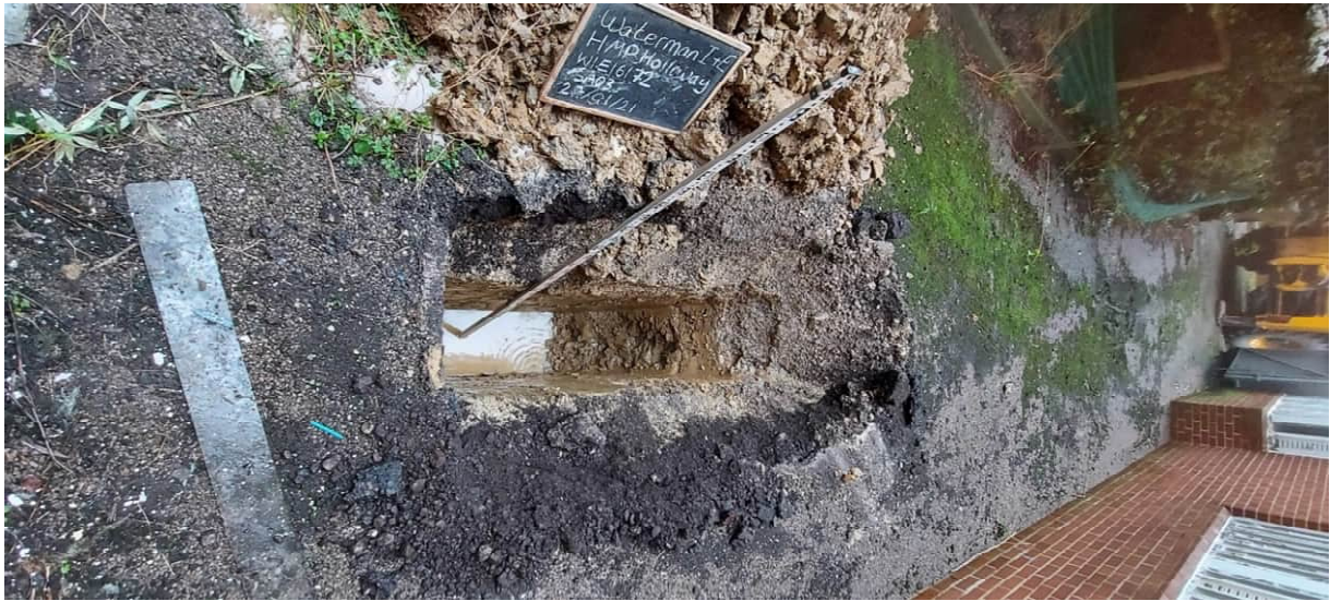
Photograph 7 – SA03 with the water ingress from the shallow made ground soils.
