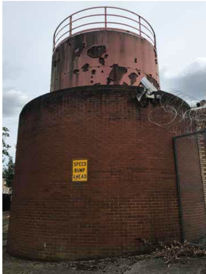
151,370 litre diesel tank
