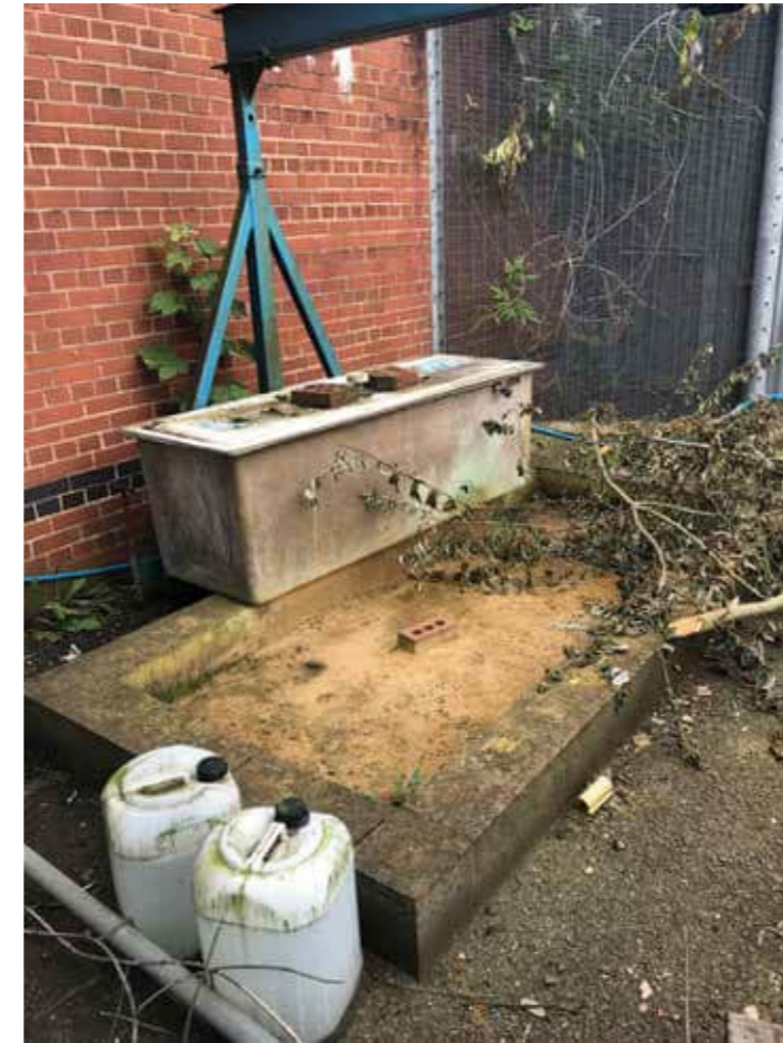
Boiler house chimney stack. Hazardous substance storage in yellow bund.
