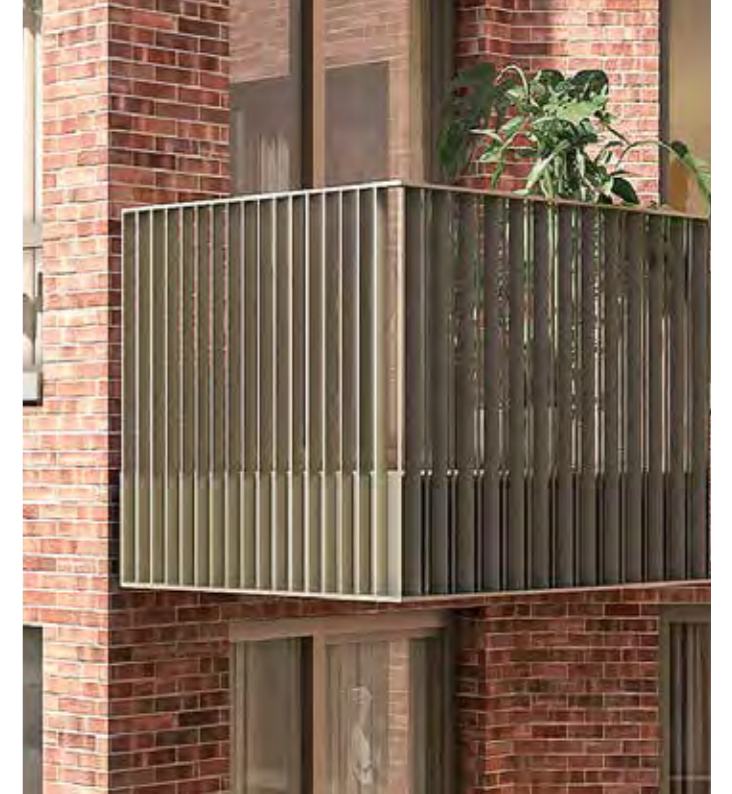
■ Painted metal guarding with angled metal flats for privacy and painted metal handrail and soffit
